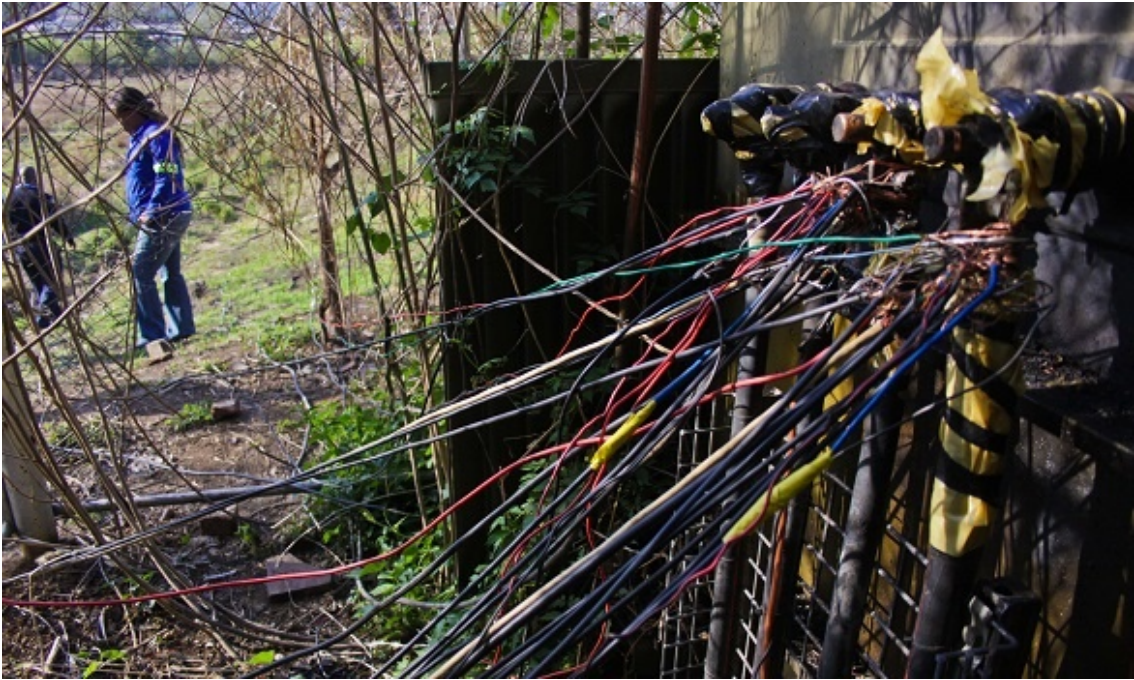
Bootlegged electricity – informal wiring
